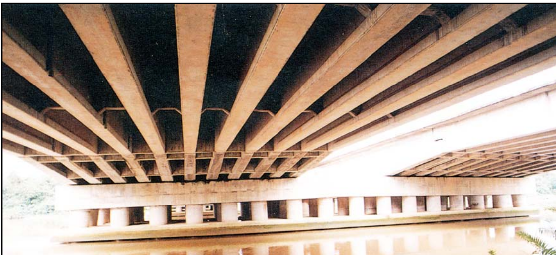
334 metres long dual-lane highway Precast Prestressed Concrete Girder Bridge over Sg. Muar,
