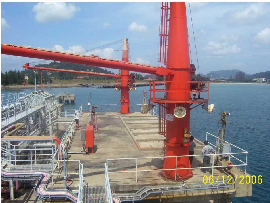
Upgrading of The Existing Liquid Chemical Berth (Lcb) Jetty at Kemaman Port
