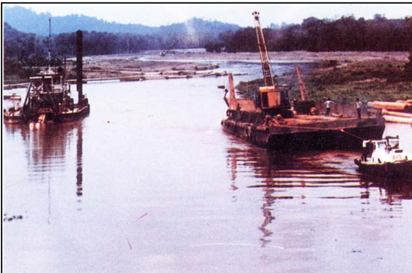
Dredging works at upstream of Parit Sulong Bridge with cutter suction, dredger and connected pipeline for spoil disposal at bunded designated area
