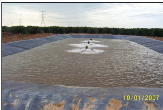
Preliminary Aeration in Leachate Pond
