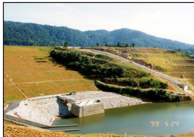
Diversion tunnel outfall structure on the left; 20m high pumping station in the centre; and 240m long spillway in the background
