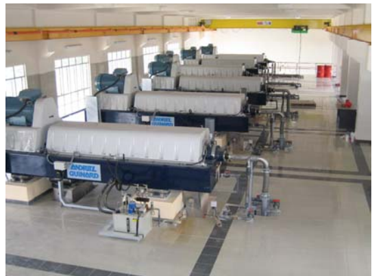
SLUDGE DEWATERING CENTRIFUGES
