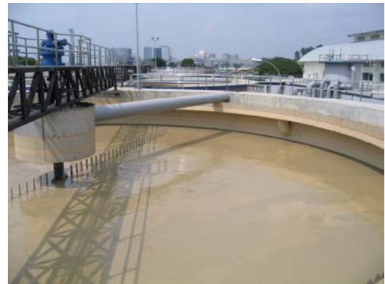
GRAVITY SLUDGE THICKENERS
