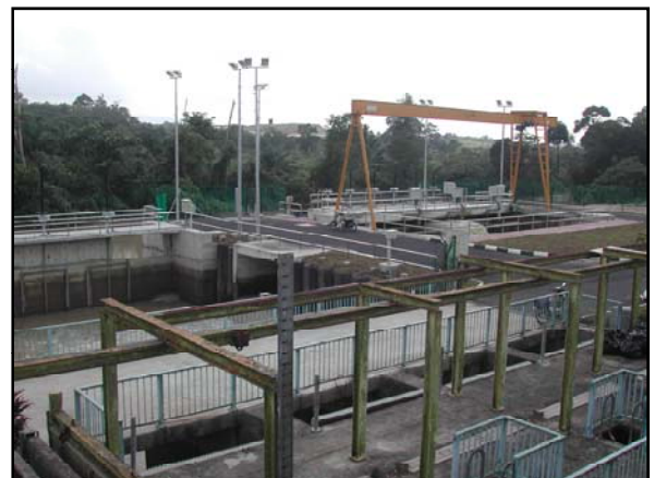
SG. JOHOR RAW WATER INTAKE
