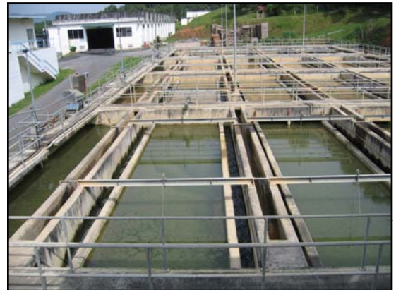
SLUDGE BLANKET CLARIFIERS
