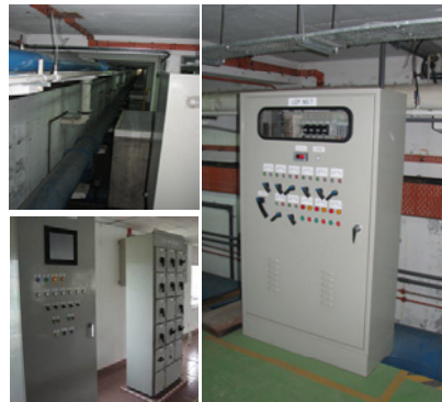
Control System for Automation Backwash
