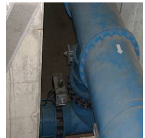
Filter backwash valves and piping systems
