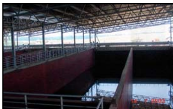
View of Aeration Tank
