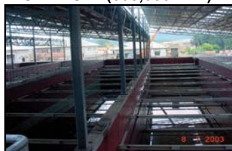
View of Final Settlement Tank
