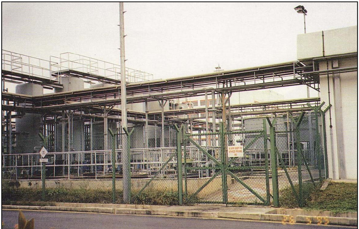
Mas Industrial Waster Water Treatment Plant
