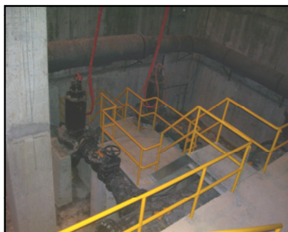
SEWAGE PUMPS AND PIPING WORKS
