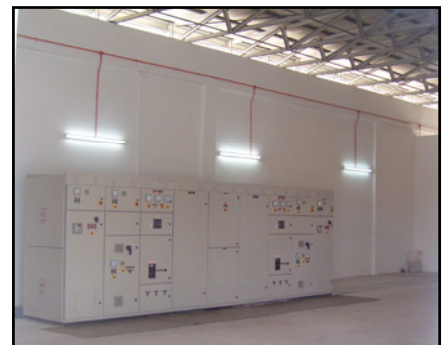
Motor Control Panel
