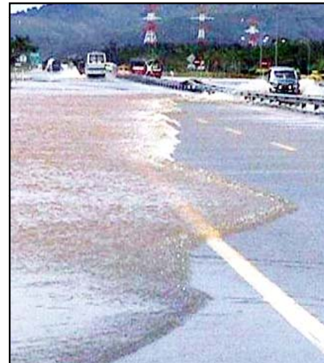
North – South Expressway - inundated during 1999 flood
