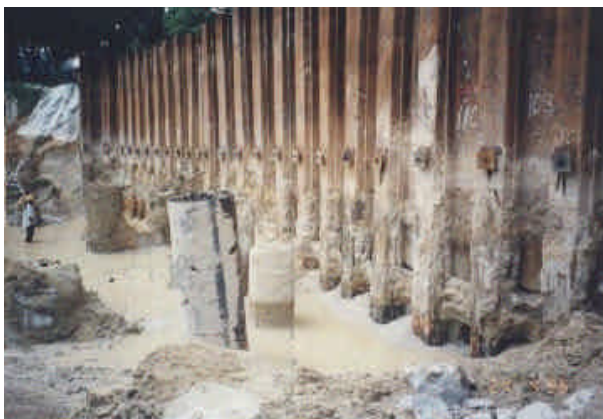
Figure 2 : The Installed Jack-In-Pipe Anchorages at the Sheet Pile Retaining Wall of 9m High
