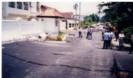
Fig. 10 A sinkhole at Jalan Lidcole (GESB 1995)
