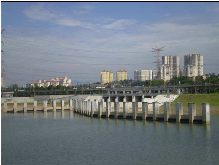
Figure 4: The Holding Pond: Baffle Walls with the Sg Klang Offtake Structure in the Background
